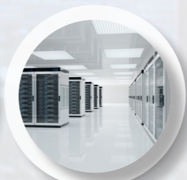
Small Data Centre (Backup purpose)
