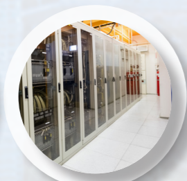
Office Server Rooms
